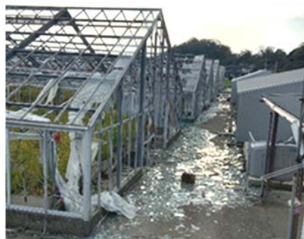
Damaged glass greenhouses (Typhoon Faxai)
